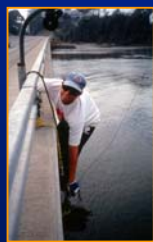
SJSU graduate student Chris Malzone installs an S4 current meter off the New 1 bridge at the mouth of the slough.
